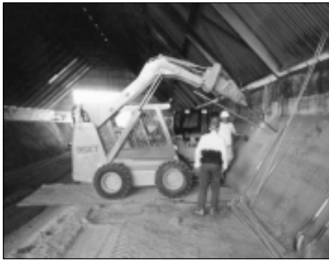
Driving MANTA RAY anchor with skid steer loader. Note small bench and new steep slope. Old slope and floor are visible at left side of photo.
